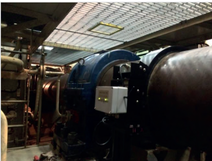
[SPECS Torque Power Meter is installed at vessel]
